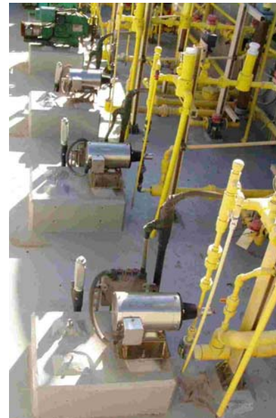
Vallejo Sanitation: 12.5% Sodium Hypochlorite metering: Tuthill D-Series pumps replaced diaphragm pumps
